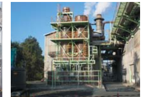
Exhaust gas scrubber
