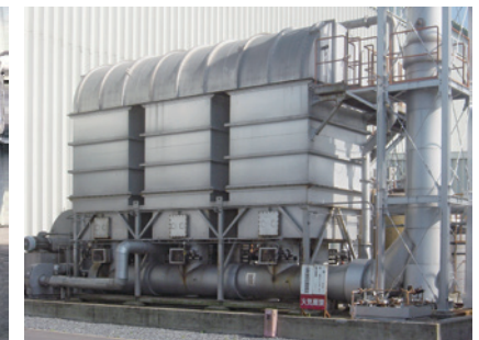
Regenerative thermal deodorizers
